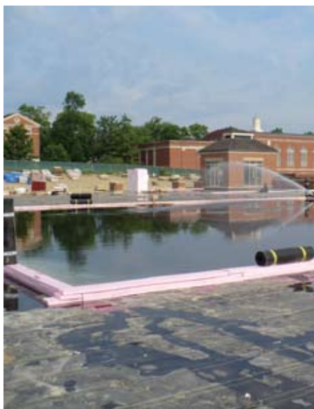
Figure 4: Plaza level waterproofing being tested before placing soil and landscape. Photo by THP.
